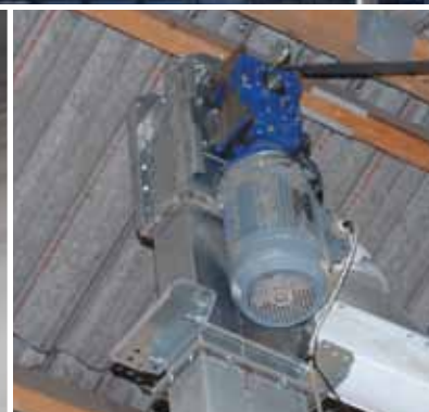
Elevator head with gear motor.
