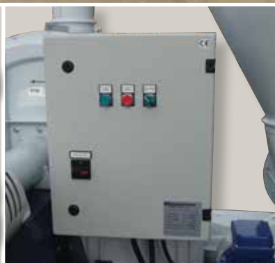
Control cabinet for automatic starting/stopping the motor.
