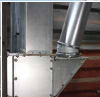
Elevator boot inlet.
