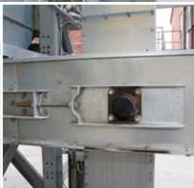
Return section with equipment for tensioning of conveying chain.
