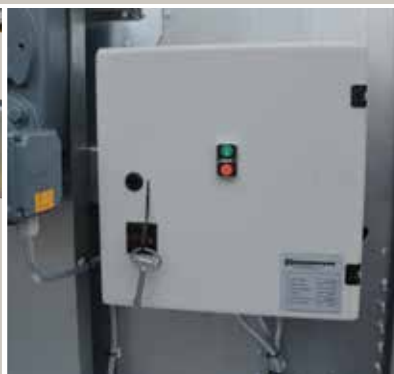
Panel for start and stop of motors in sequence, only one power supply wire is required.
